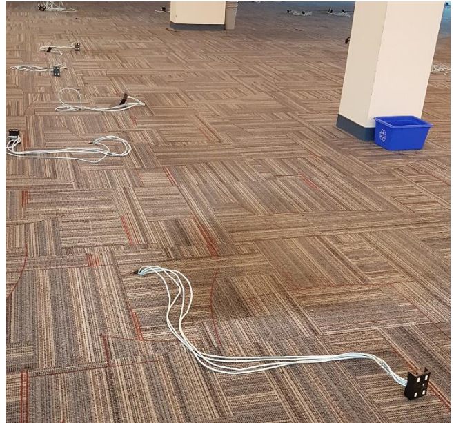
Figure B - Sample of staining and cord management through carpeting
