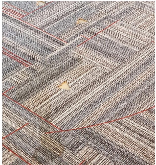
Figure D – Excess holes in carpet from power feed placement
